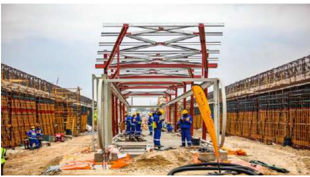
A construction site of the Rea Vaya route in Johannesburg. (Photo by Sharon Seretlo/Gallo Images via Getty Images)
